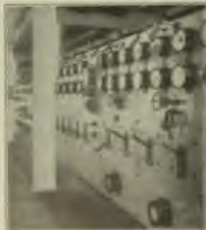
FIG. 14. MAIN ALTERNATING-CURRENT SWITCHBOARD
